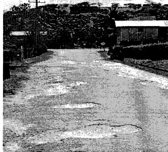
Picture 3: Inadequate municipal road maintenance in Santa Elena
