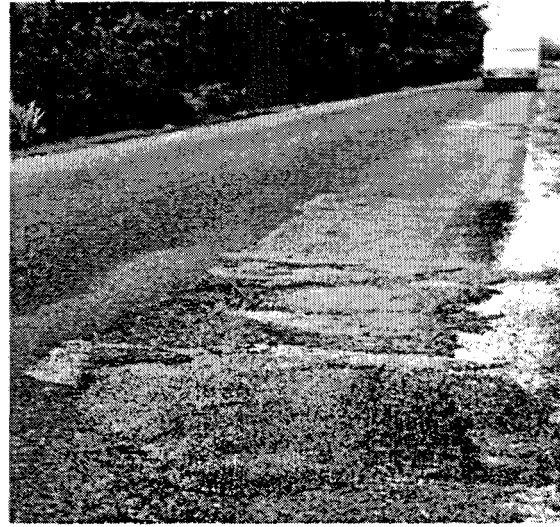
Picture 5: Patch maintenance is the norm – the main Northern Highway between Belize City and the international airport
