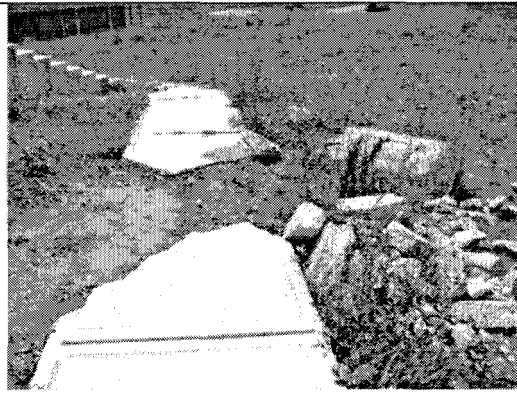
Figure 3.5: Poorly constructed concrete
