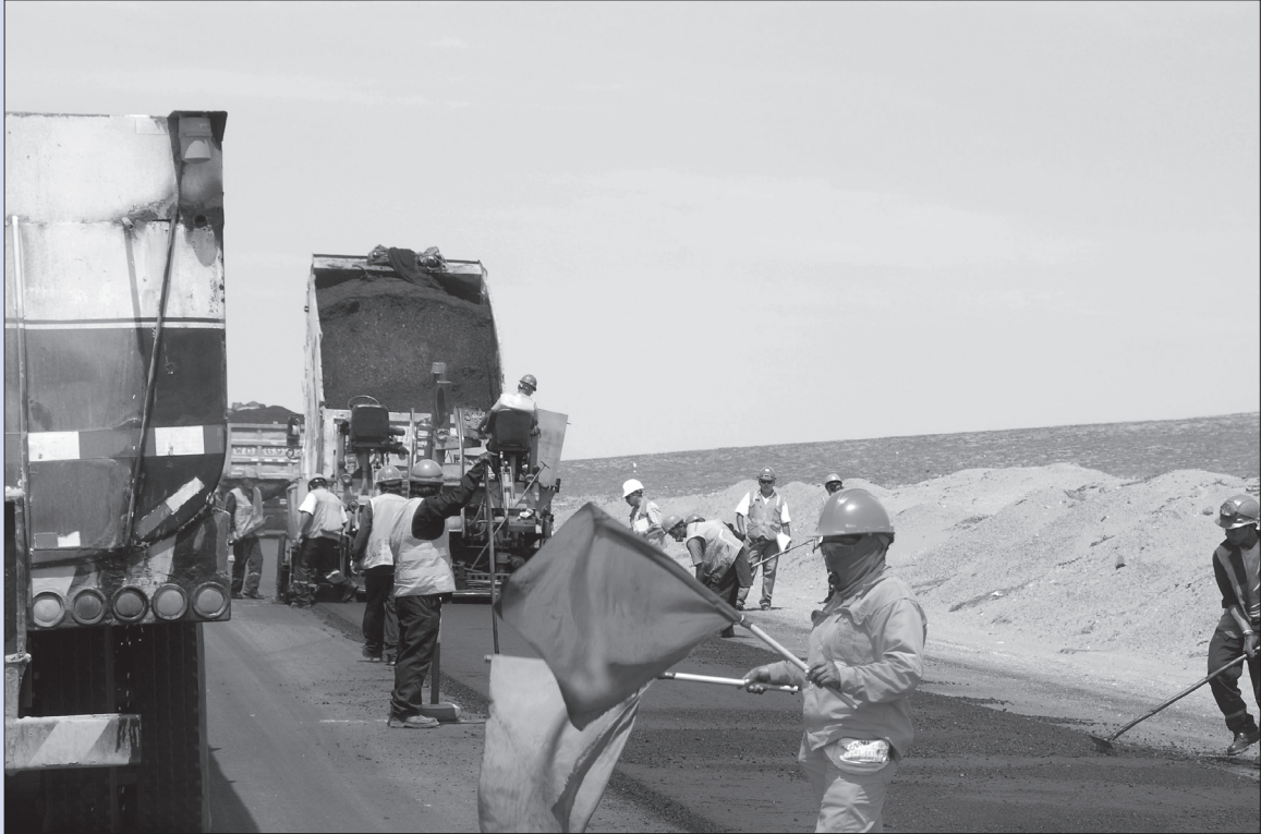
Crews working on a road in Peru. Photo courtesy of Jouni Martti Eerikainen.
