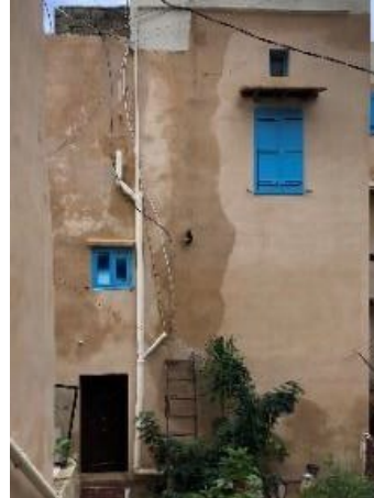
Figure 3.2. Water Leaks through CHUD-Installed Works
