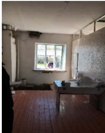
The health center undergoing replacement of windows to allow for more light to enter
